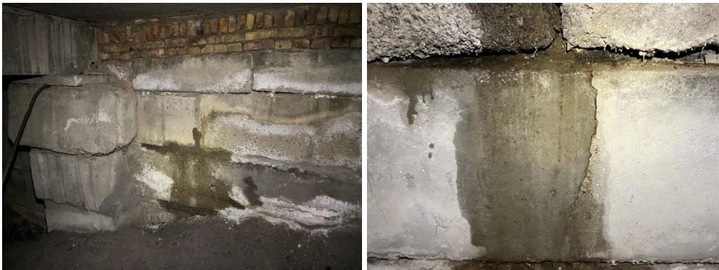
Figure 2 – Efflorescence (left) and shrinkage cracks (right) of foundation
