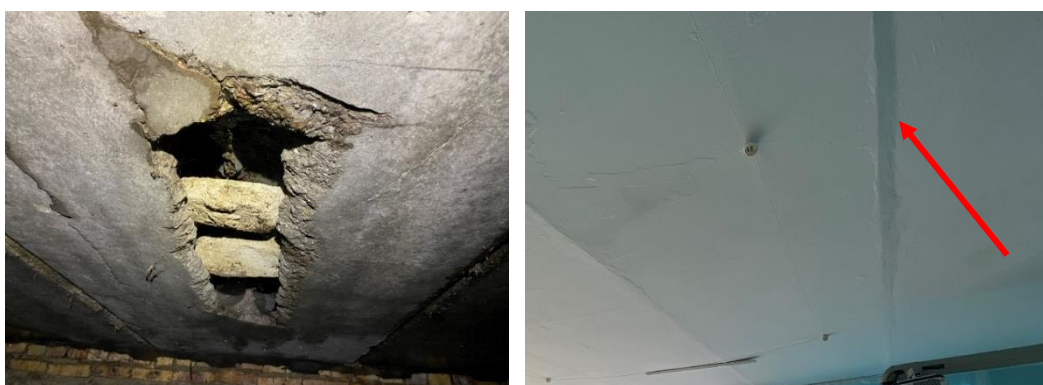
Figure 6 – Breaks (left) and displacement (right) of slabs
