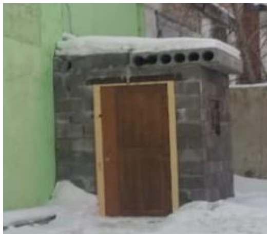
Figure 10 – Full-scale tests of the manufactured pilot-industrial batch of products «Hollow wall stone with ash-and-slag waste» in the form of construction of an extension to the production workshop of EcostroyNII-PV LLP
