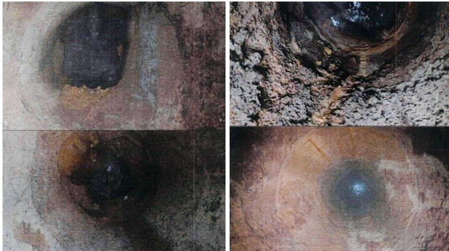
Figure 2 – Pipelines condition before CIPP installation
