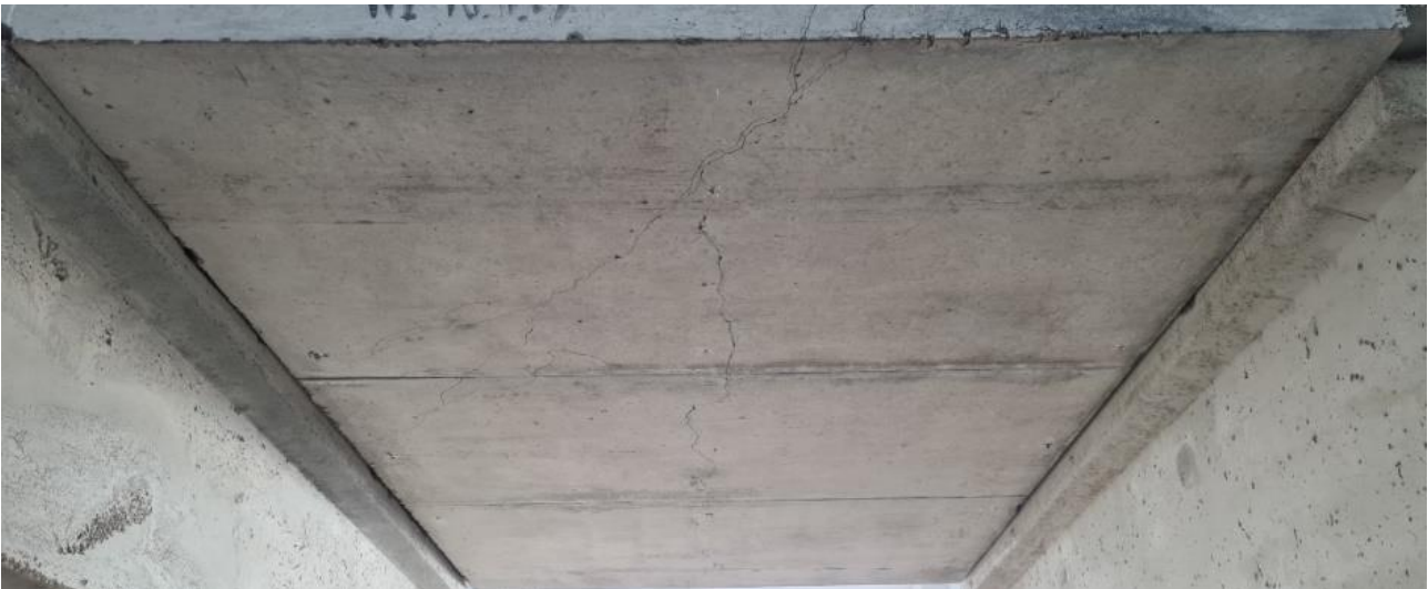
Figure 14 – Cracks in the interlocking floor slab
