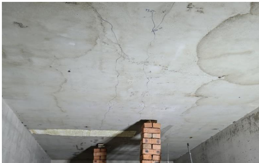
Figure 12 – Cracks in the ceiling slab
