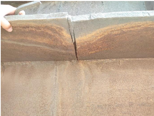
Figure 8 – Support ring of gas outlet shaft No.1 at the level of site level at level +49.200
