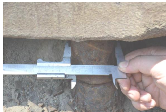
Figure 4 – Continuous irregular corrosion of foundation bolts
