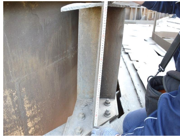
Figure 9 – Rolls and loss of local stability of the walls of the support beams of gas outlet shafts characteristic for beams at the site level at level +49.200
