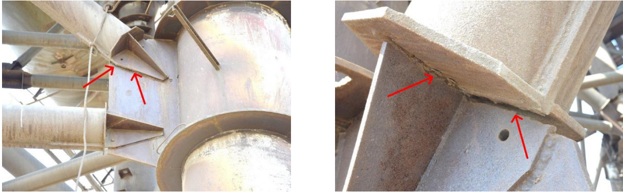
Figure 5 – Characteristic critical defect: weld rupture in the connection between the strut attachment plate and the fascia
