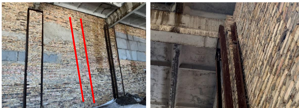
Figure 3 – Weak bonding (left) and poor strengthening (right) of masonry
