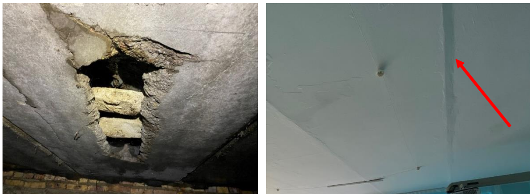
Figure 6 – Breaks (left) and displacement (right) of slabs
