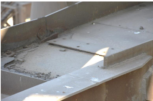
Figure 6 – Fracture of the weld along the entire length of the joint
