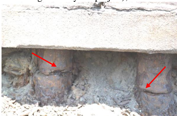
Figure 3 – Breakage of foundation bolts
