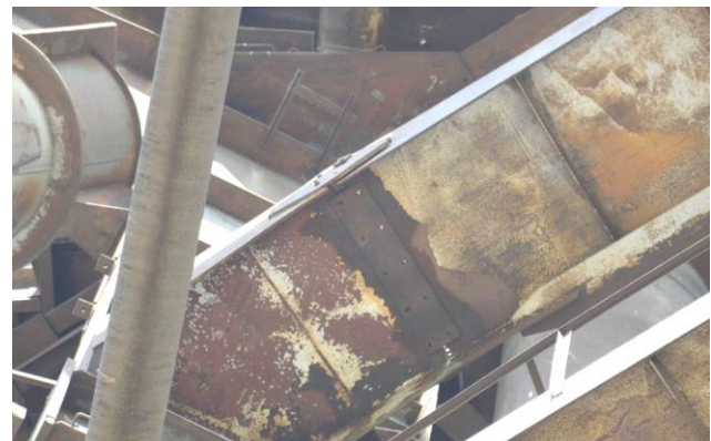
Figure 7 – Fracture of the weld at the fusion boundary along the entire length of the joint
