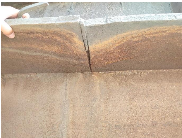
Figure 8 – Support ring of gas outlet shaft No.1 at the level of site level at level +49.200
