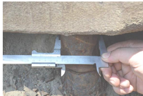
Figure 4 – Continuous irregular corrosion of foundation bolts
