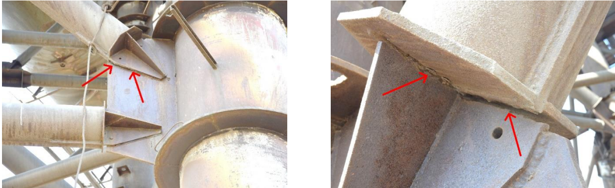
Figure 5 – Characteristic critical defect: weld rupture in the connection between the strut attachment plate and the fascia
