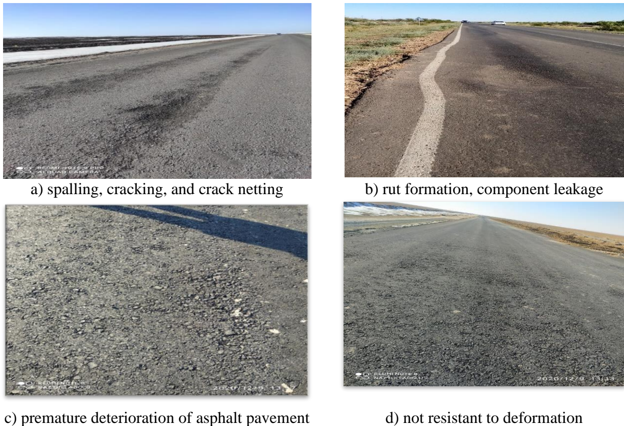
Figure 1 – Types of pavement failures [12]
