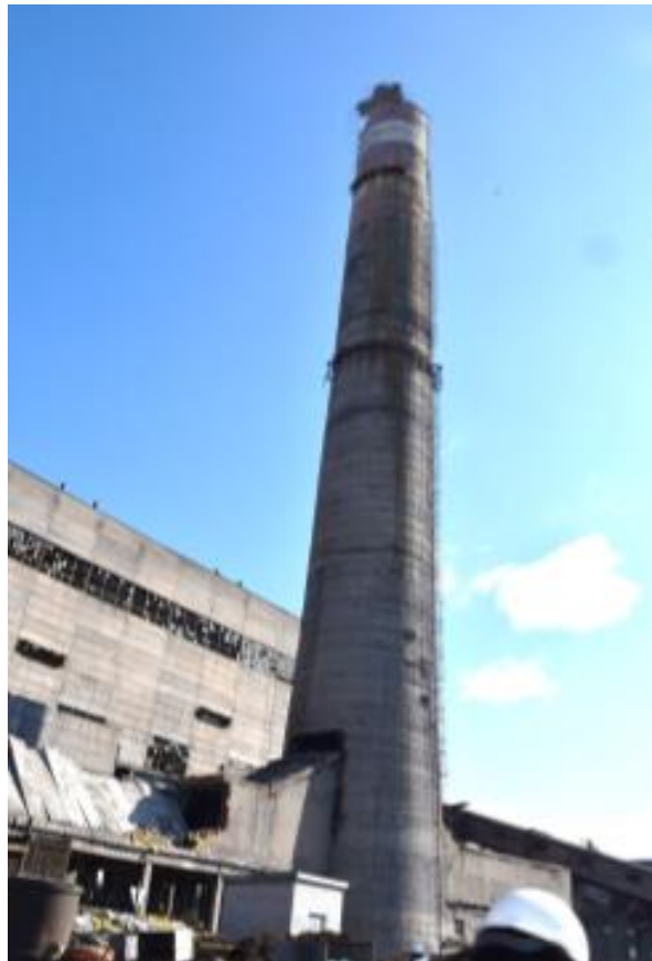
Figure 1 - General view of the chimney of Petropavlovsk TPP-2 after collapse
