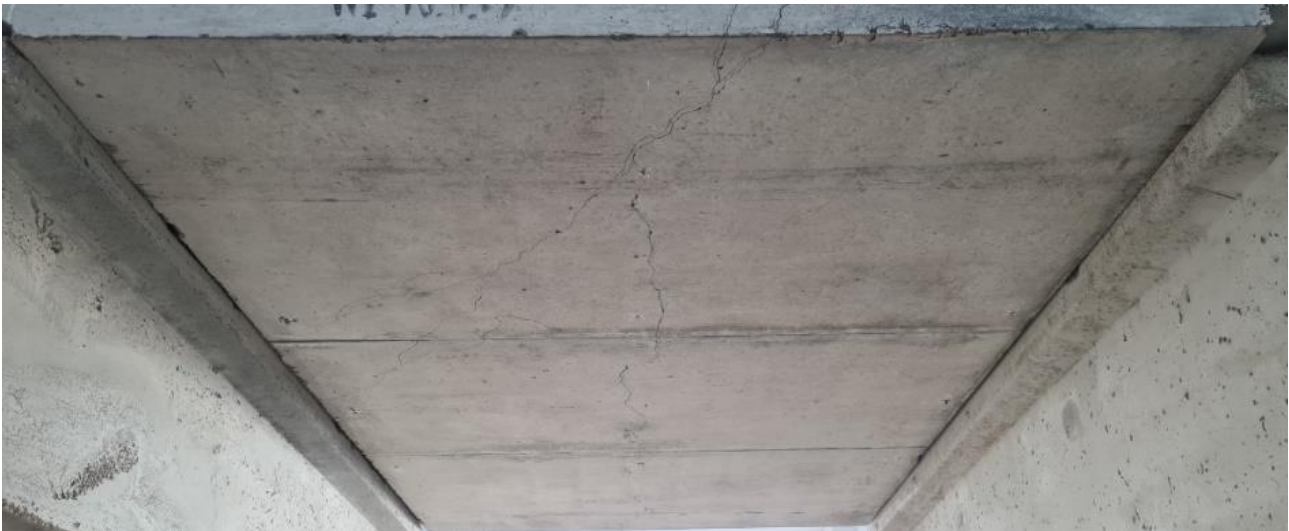
Figure 14 – Cracks in the interlocking floor slab
